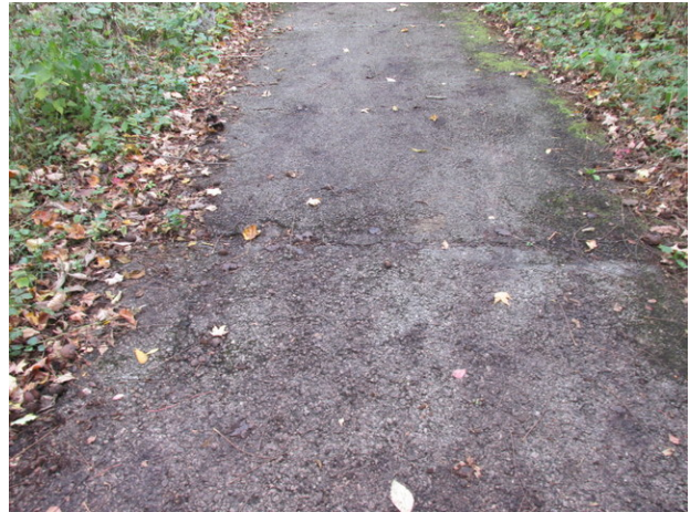
Asphalt walking path deterioration
