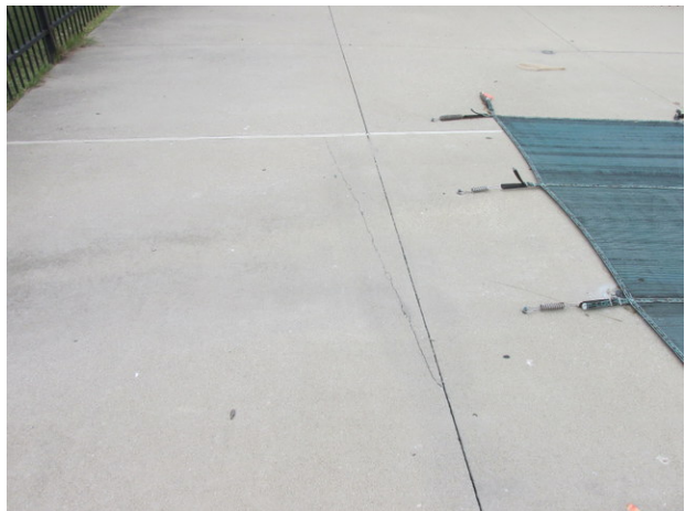
Isolated concrete deck crack
