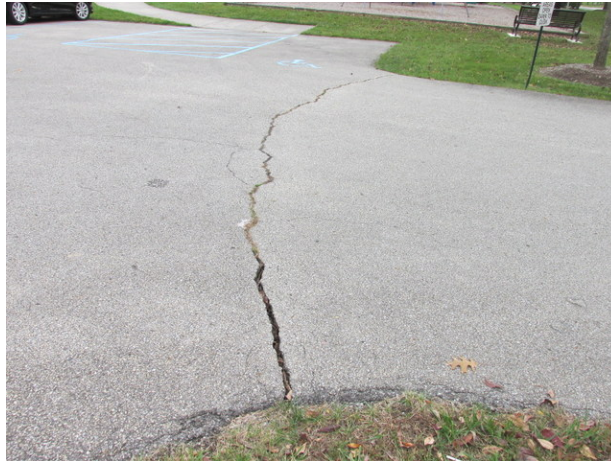
Asphalt pavement crack
