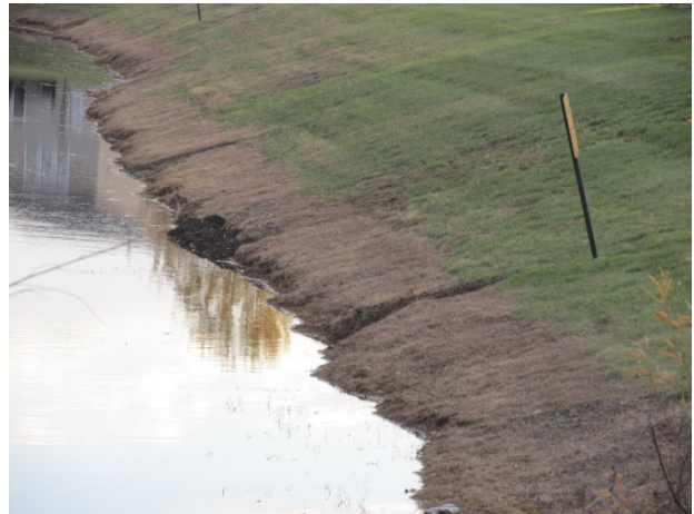
Minor erosion at pond off of Memorial Knoll Drive
