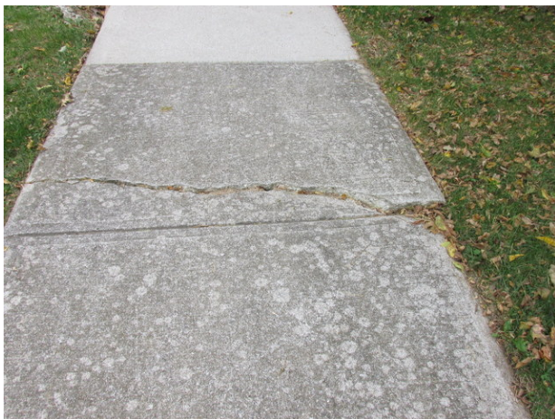
Concrete sidewalk crack and trip hazard
