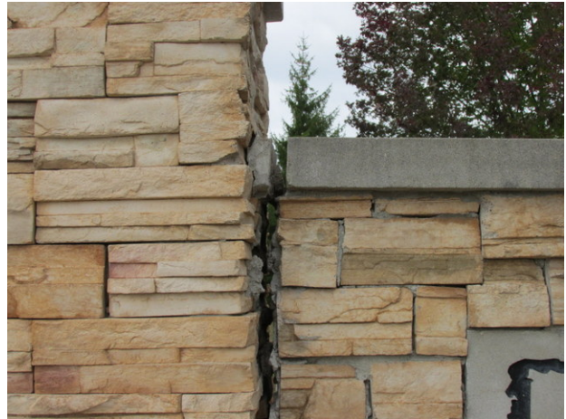
Settlement of the masonry at the Tallgrass community entrance
