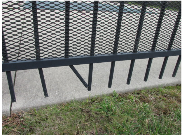
Isolated damage at the Tallgrass community pool fence
