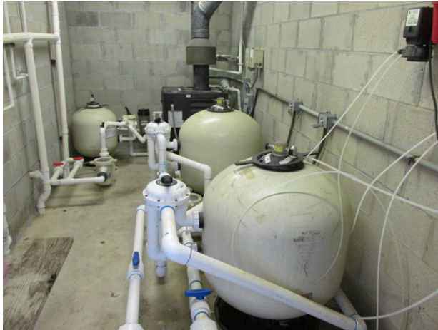
Pool mechanical equipment
