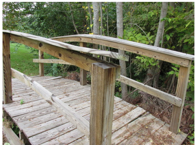
Deterioration of railing and deck boards
