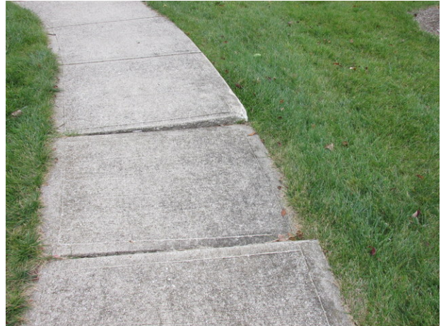
Isolated trip hazard
