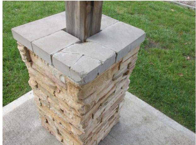
Isolated cracked cap at masonry column base
