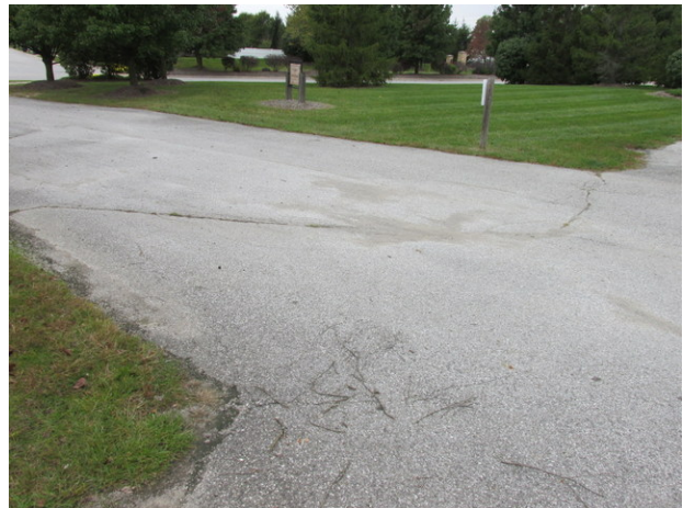
Asphalt pavement crack
