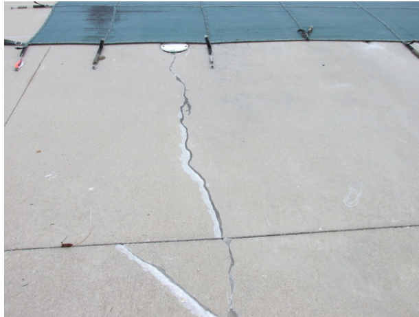
Evidence of previous crack repair at deck
