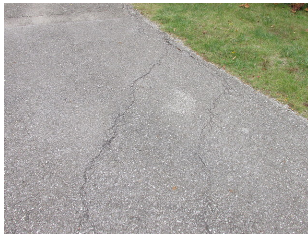
Asphalt walking path cracks
