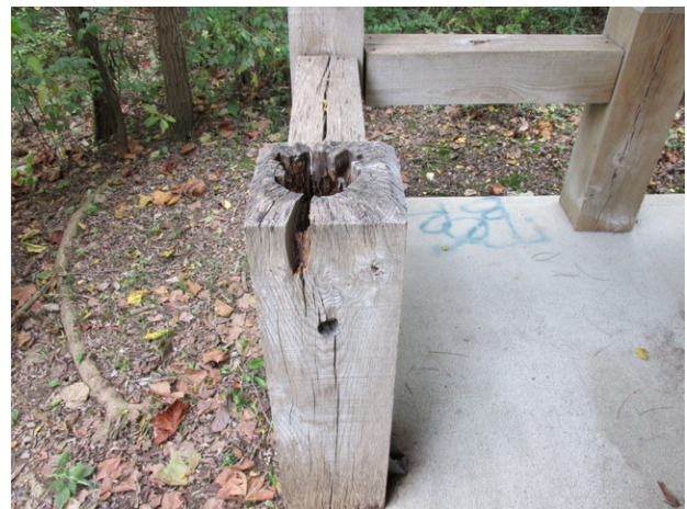
Railing post deterioration
