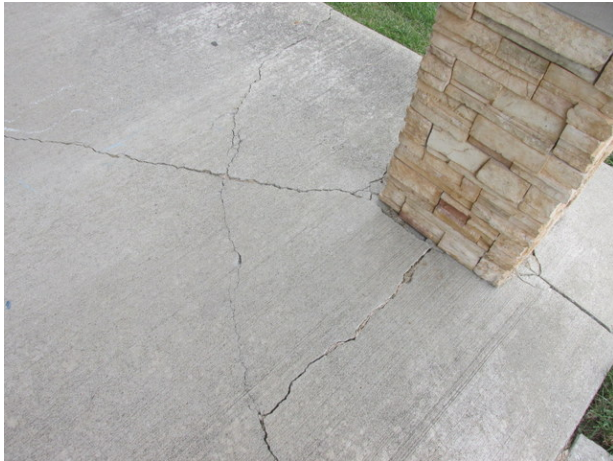
Concrete cracks at pavilion
