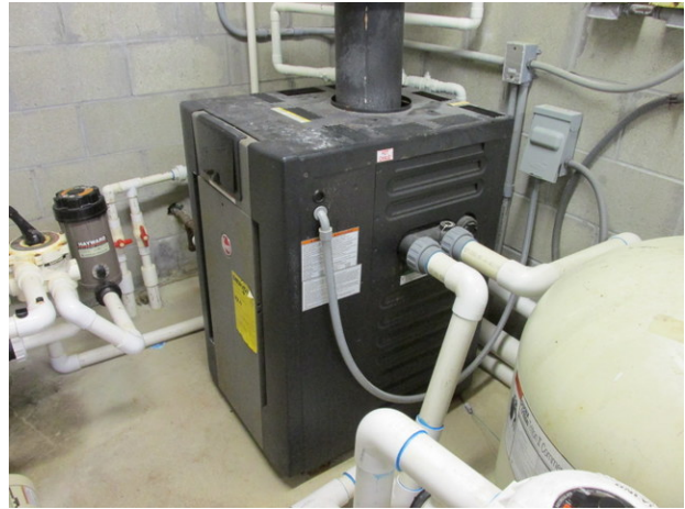
Pool water heater
